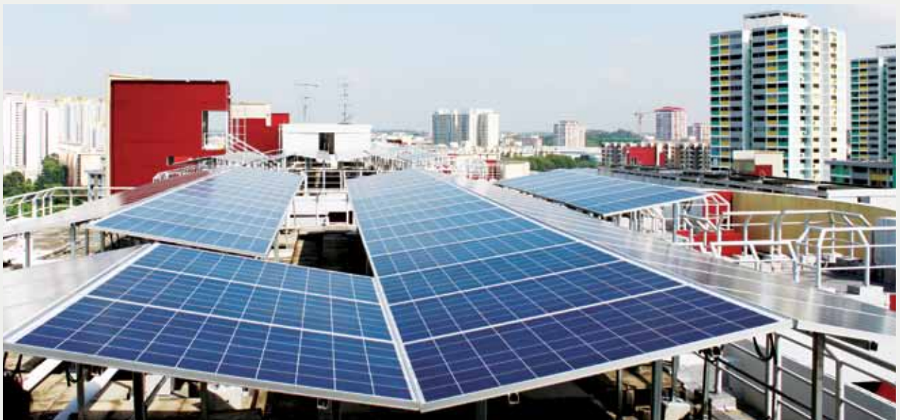
Solar panels on a public housing block at Jurong East Street 24.
