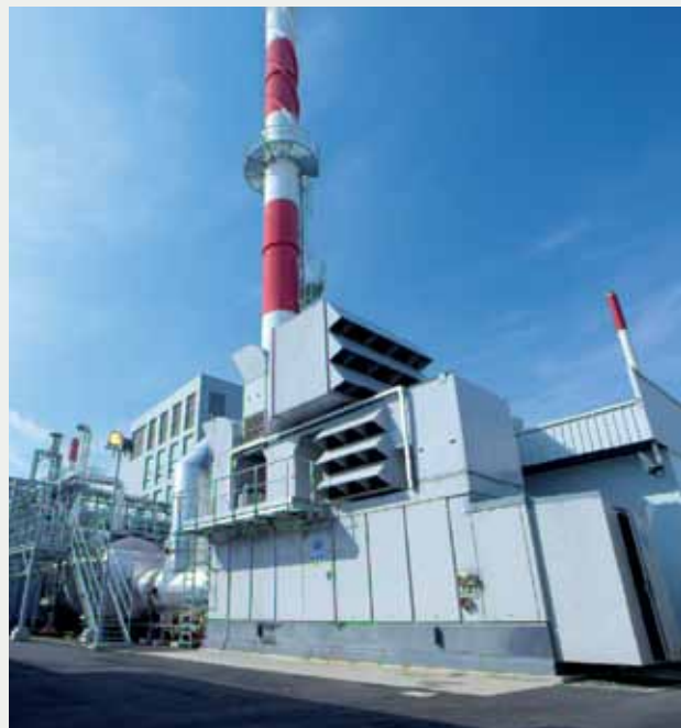
First Trigeneration plant in Singapore, owned by Pfizer Asia Pacific and developed by TPGS Green Energy.
