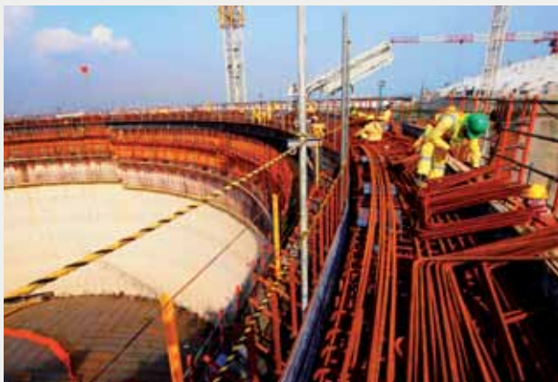
Singapore's first LNG terminal in Jurong Island, scheduled to be completed in 2013.
